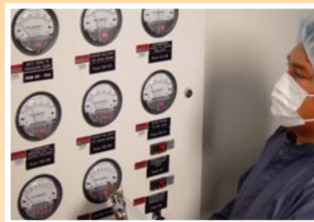
Air pressure is maintained in our production core so that air flows from critical areas to less critical areas.
